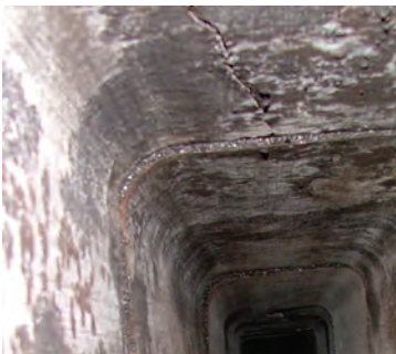
Cracked flue tile
