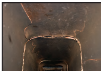
Actual photo of cracked flue tiles
